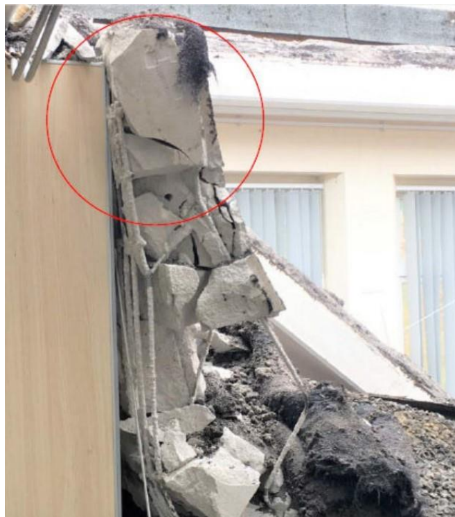
Figure 2: 2018 Roof Slab Collapsing (SCOSS)
