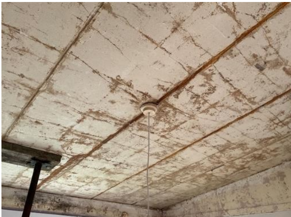
Figure 6: Typical RAAC panels condition observed during surveys
