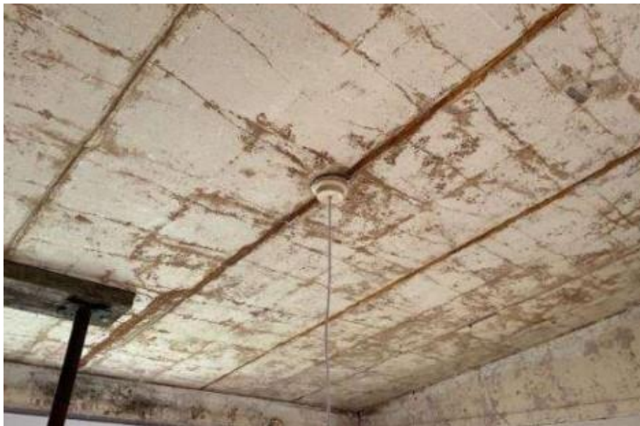
Figure 5: Typical RAAC Panel Condition observed from surveys
